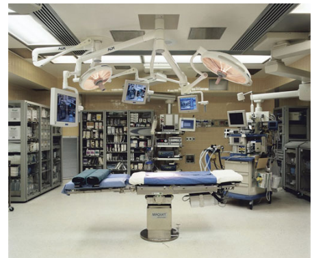
Figure 5. Surgery / Clean Room
